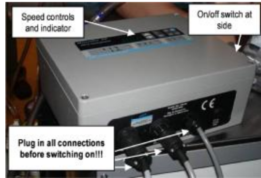
Figure 3.16: circuit pump control unit
